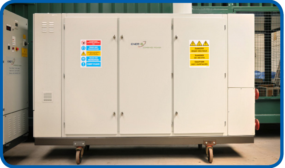
Internal CHP unit at St Ambrose College designed by ENER-G
