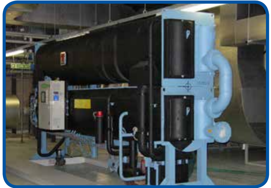
ENER-G's CHP system at Royal Shrewsbury Hospital
