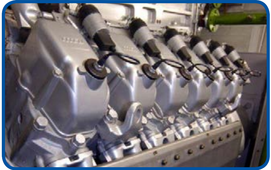
1.6 MW CHP at Loughborough University from ENER-G
