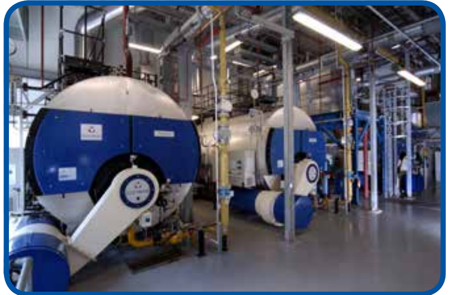
ENER-G's CHP system at Birmingham Heartlands Hospital
