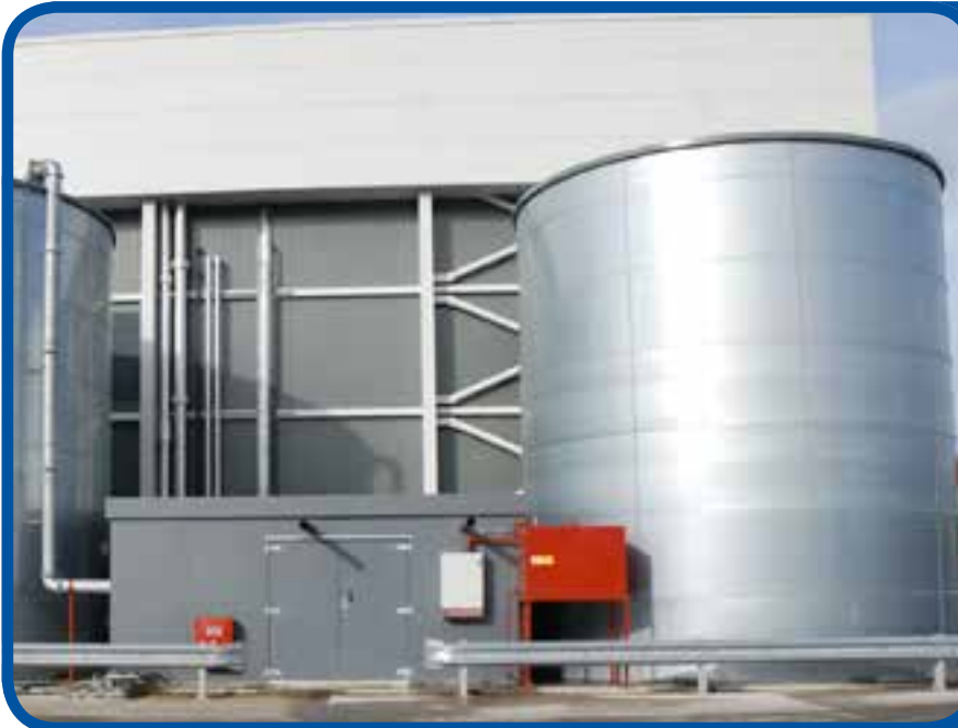
Energy centre containing the ENER-G 150 unit at Adams Foods
